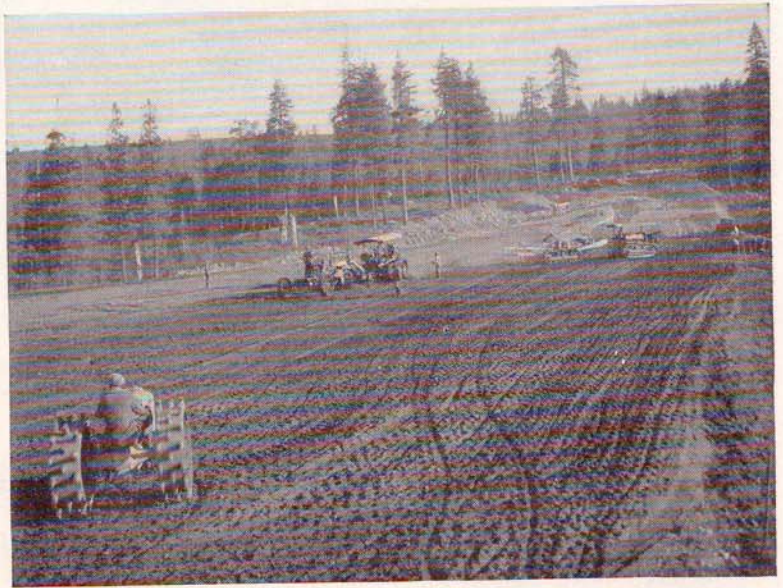
Philbrook dam under construction. Note unusual type of earth-moving machine in right background. In the foreground is a Fordson tractor, with sheep-foot tampers attached.
